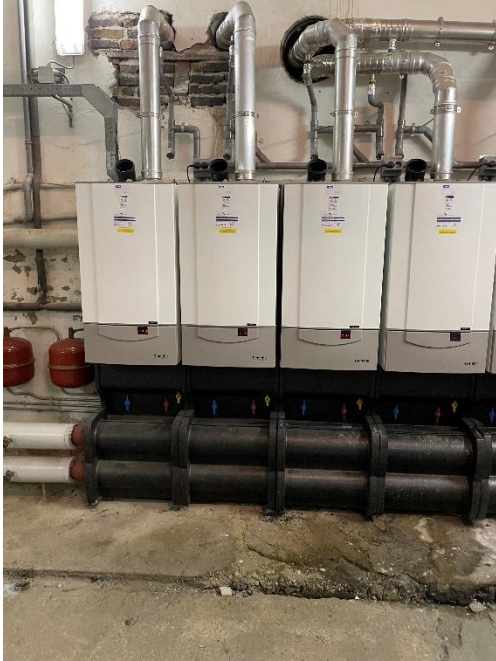
5 ketels HR 107 in cascade.
